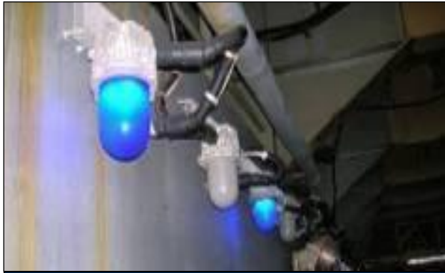
Efficient Ship Systems Example: Solid State Lighting
